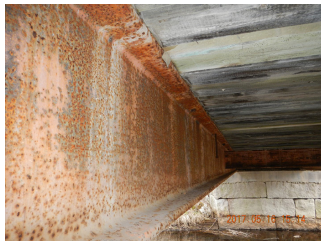
Balk ytbehandling - Korrosion.
